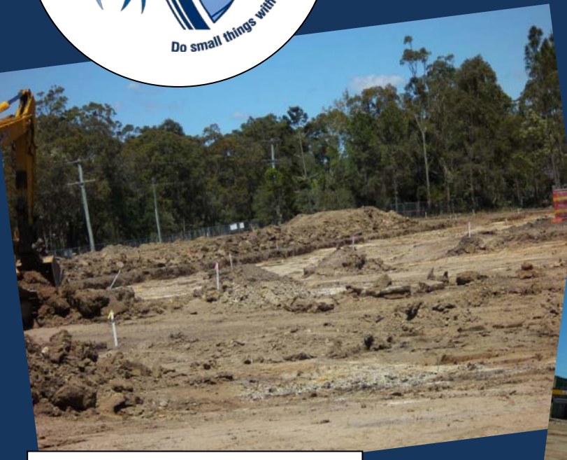
Looking South. This shows the car park and to the right of frame is the start of the administration block
